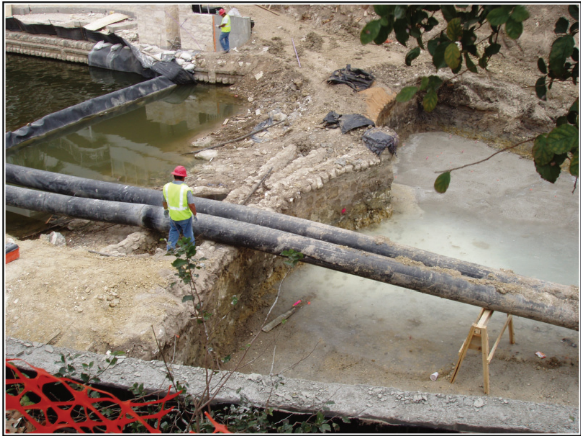
Figure 4-25. Feature 11, the Lexington Avenue Dam, prior to being cut. The feature was recorded as Site 41BX1818 during the project.
