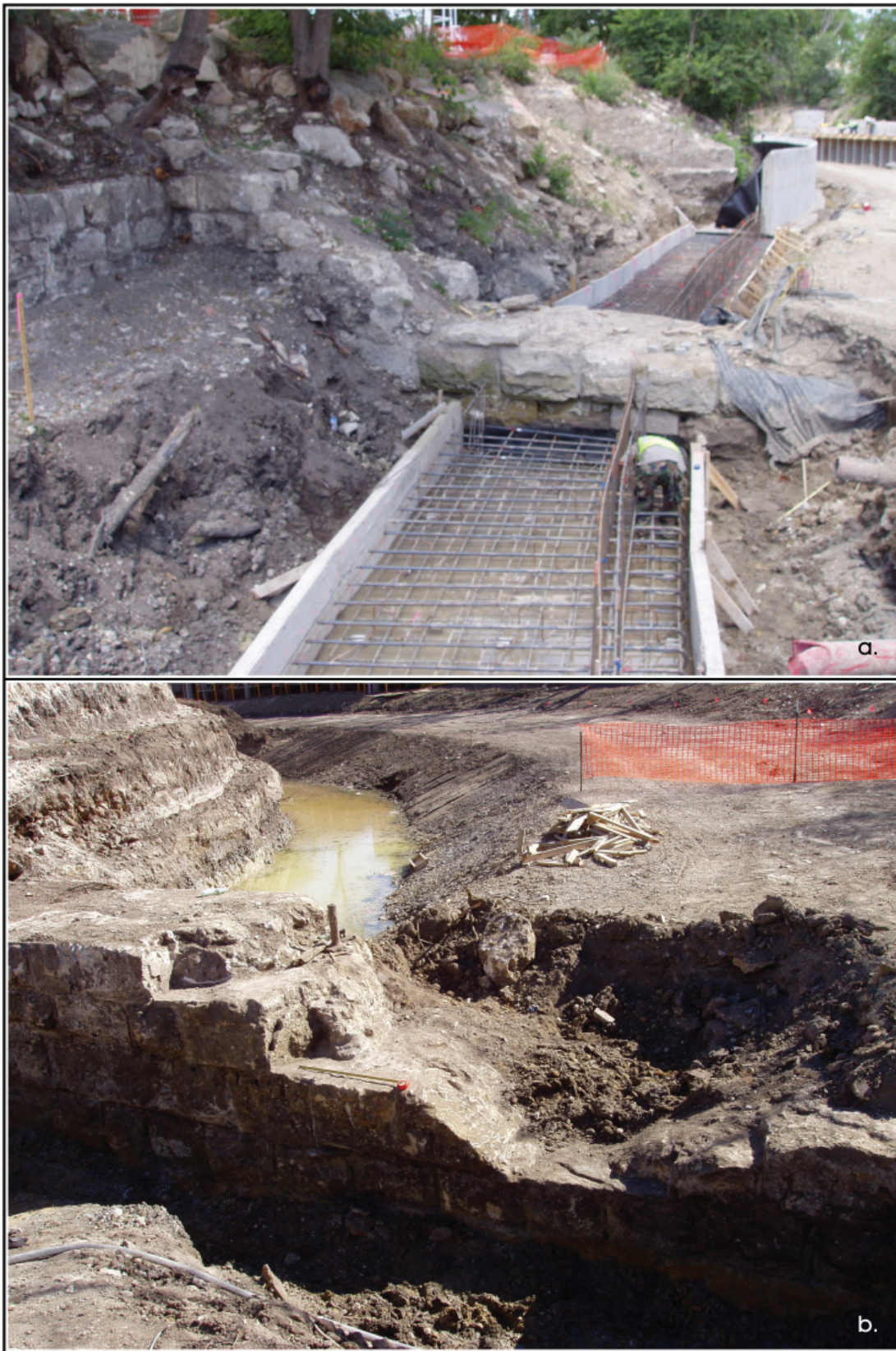
Figure 4-8. The Alamo Mills Dam after it was uncovered in 2008: a) protruding from the east bank; b) coming from the west bank.
