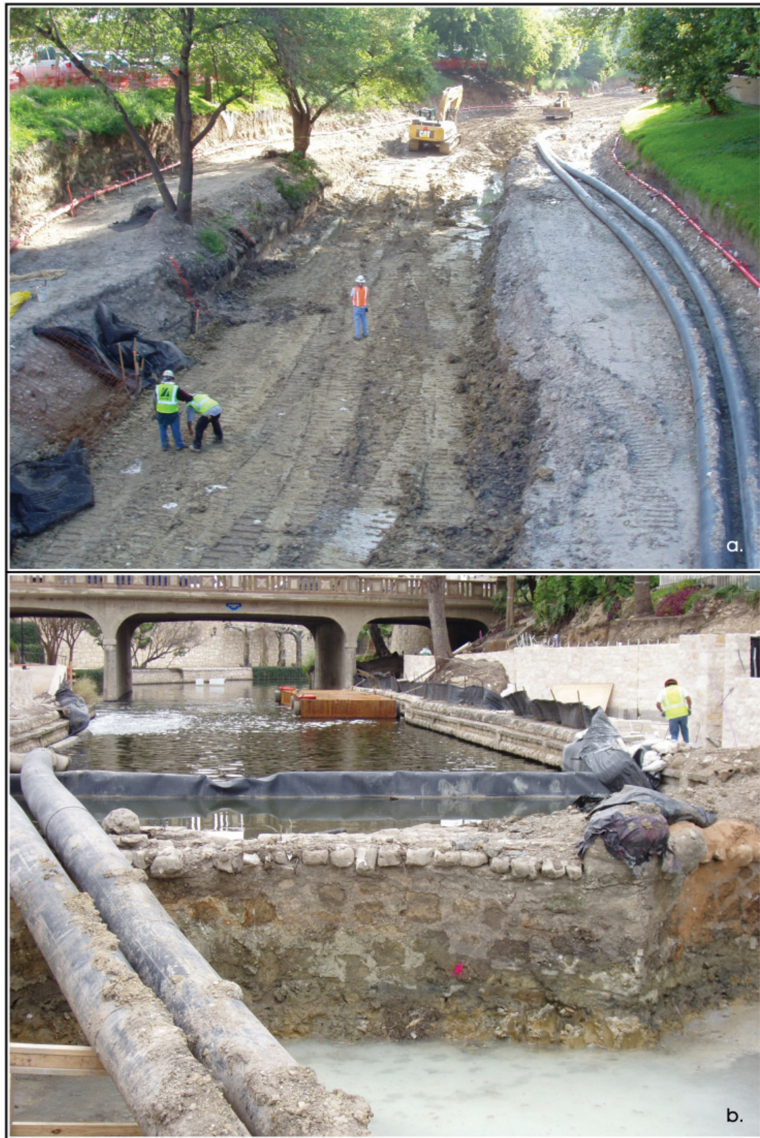
Figure 1-5. Piping river-water around the construction zone: a) river-water bypasses construction in pipes seen on the right; b) returning the water to the river at the Lexington Avenue (Hugman) Dam.
